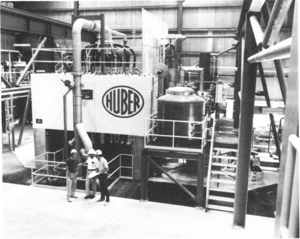
Figure 4.9. Eriez Magnetics's superconducting magnetic separator in a kaolin mill.
