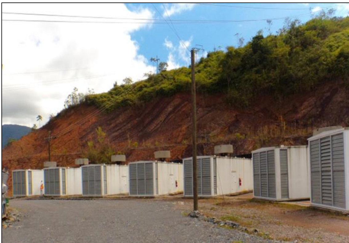
Figure 18.6 – CAT diesel generators
