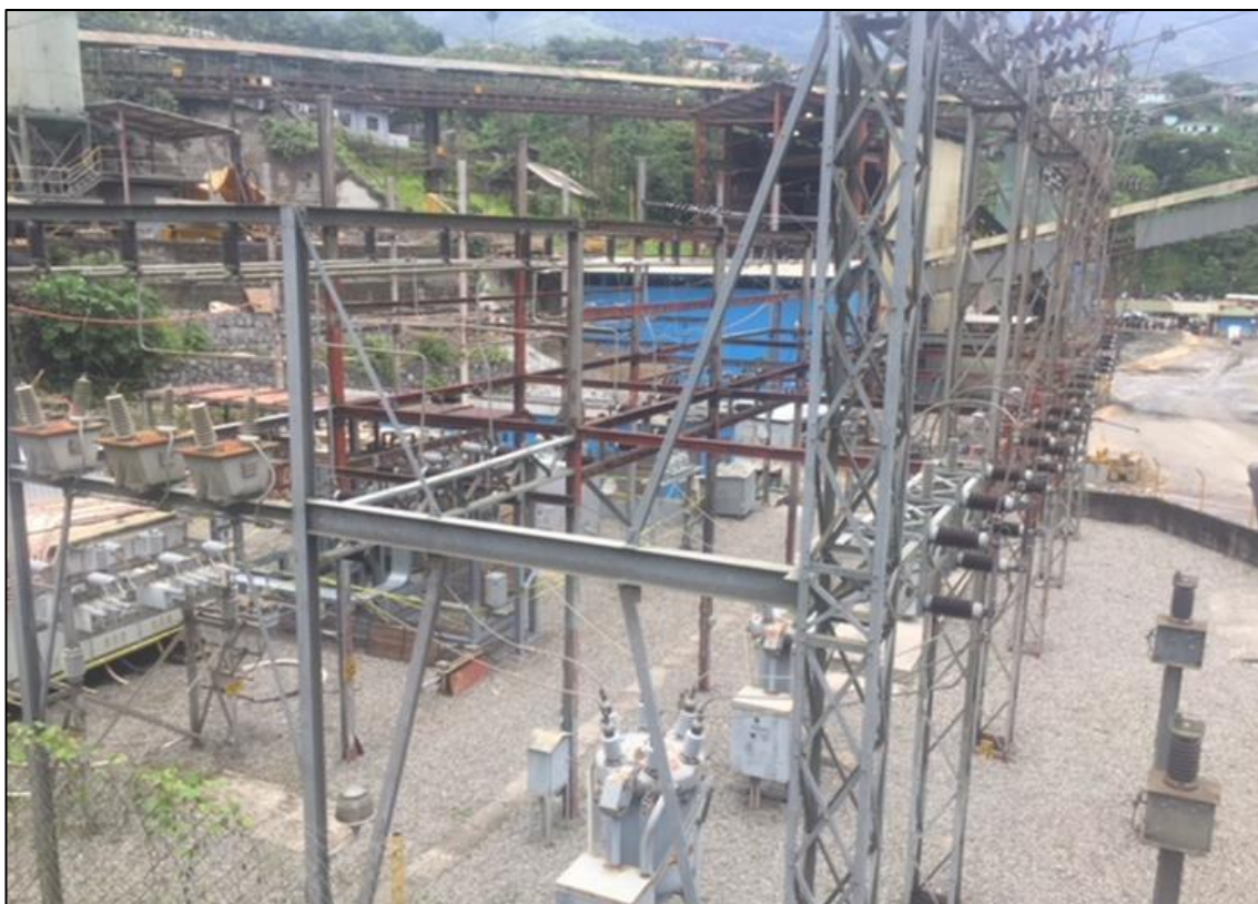
Figure 18.5 – 34.5 kV old substations
