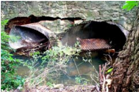
Corroded Metal Pipe
