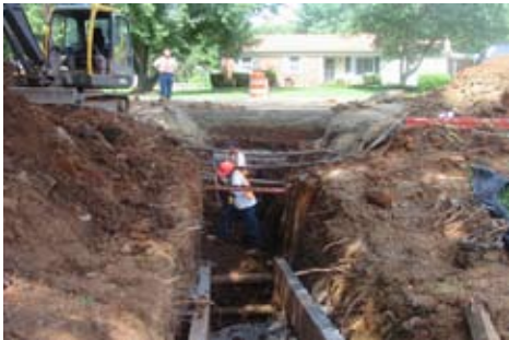
Hand Dig Utility Conflicts
