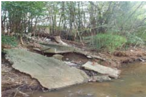
Failed Concrete Apron
