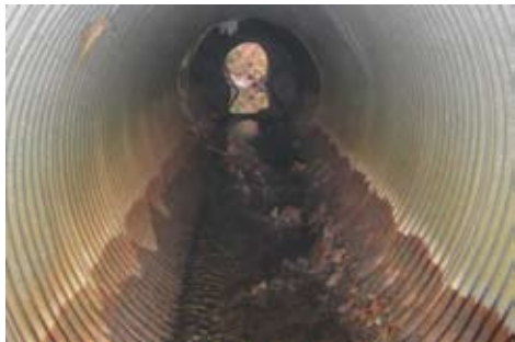
Corroded Metal Pipe
