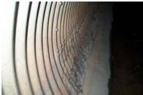
Corroded Metal Pipe
