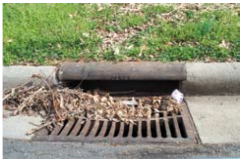
Debris at Catch Basin
