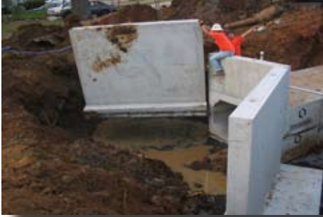
Pre-Cast Wing Wall
