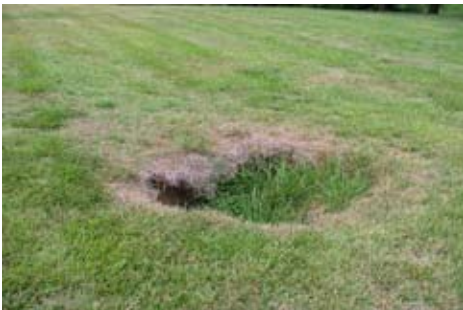
Sinkhole or Blowout
